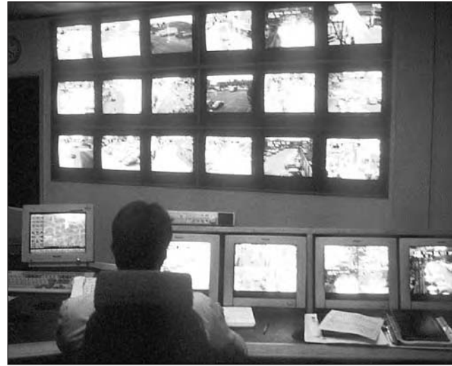
Figure 151 CCTV monitoring centre, southern England
