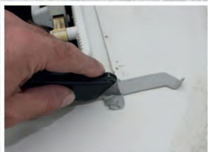
Trim the excess mastic sealing strip, taking care not to damage the roof's surface
