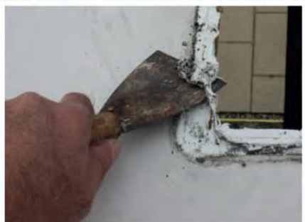
Remove the old mastic from around the edge, being careful not to damage the roof
