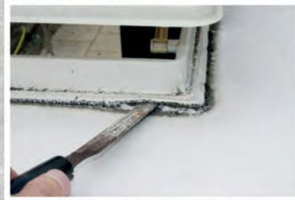
Carefully break the seal of the old mastic before taking out the assembly unit
