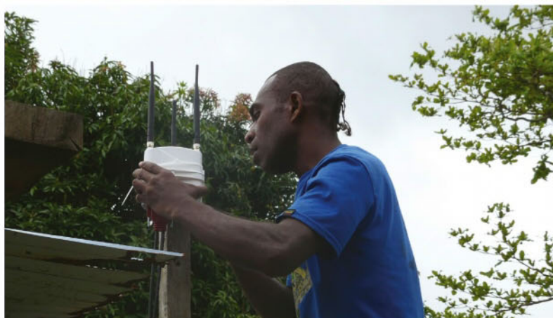
Below Installing Serval Mesh Extenders in Epau, one of the two villages targeted on the island of Efate
