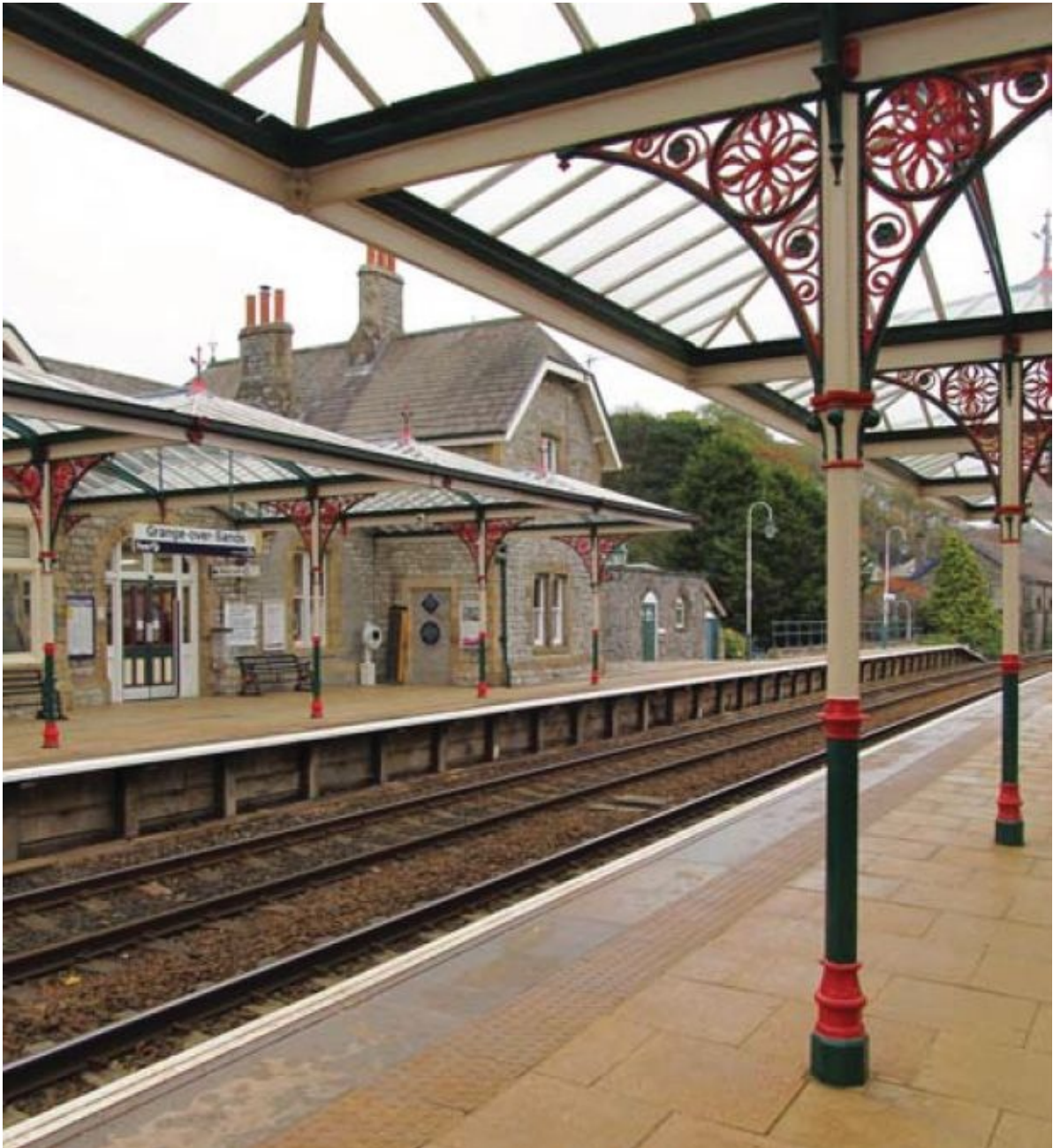
The roof at Grange-over-Sands employs standard rolled sections perched above spandrel panels of unusual delicacy. The coming of the railway established Grange as a genteel resort.
