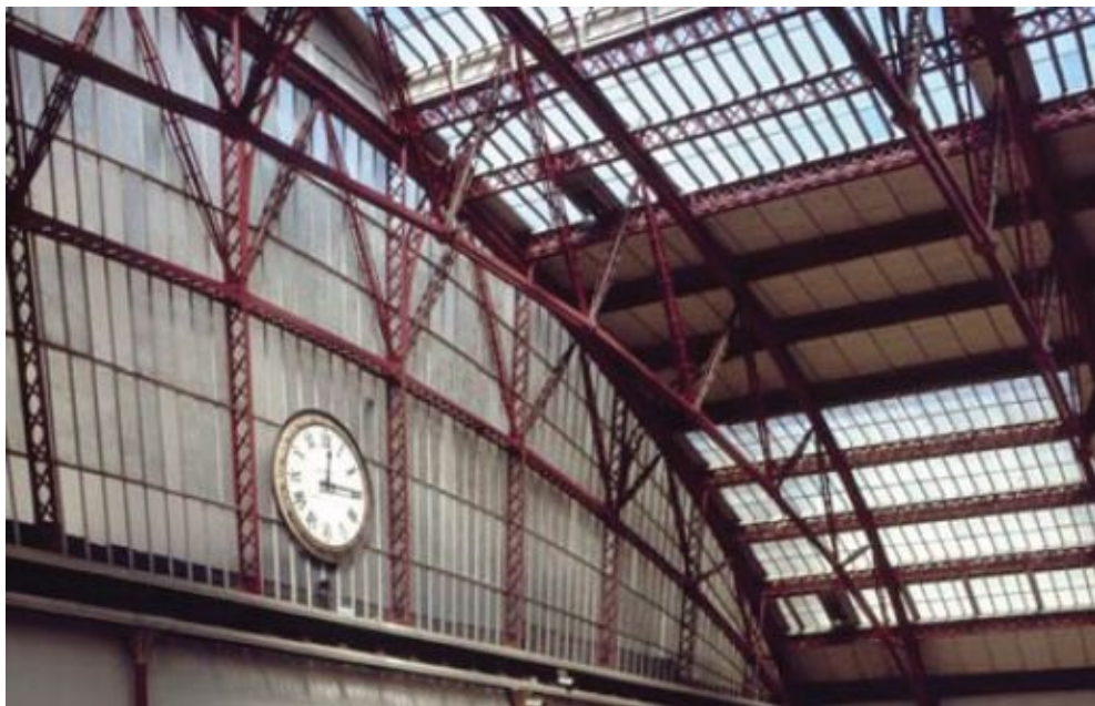
Liverpool Lime Street: 1867 span (William Baker). Though based on Cowper's Birmingham roof, the trusses are a lot sturdier and lattice girders are used for the purlins, which run lengthwise and bear the glazing, whereas Cowper had employed wooden beams.
