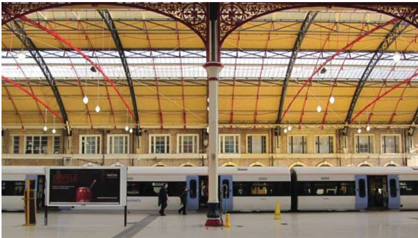
London's Victoria comprised two disparate but adjoining buildings serving different railways. This is Fowler's roof over the 'Chatham' side, which served cross-Channel trains such as the 'Golden Arrow'.
