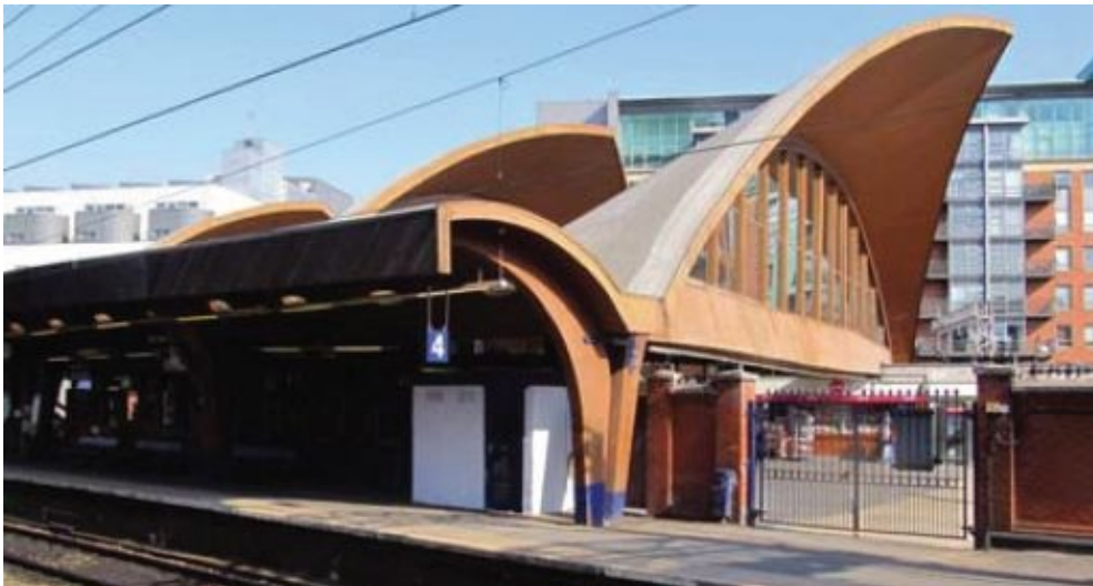
Manchester Oxford Road (Max Clendinning and Hugh Tottenham). Concealed steel reinforcement (1998) has been used to cure the onset of structural weakness.
