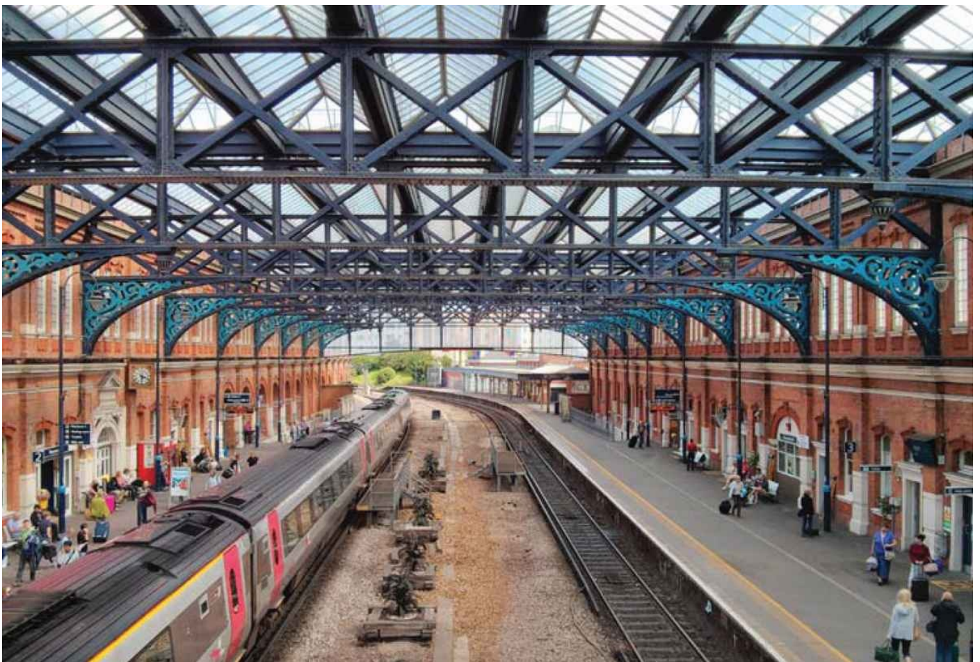
Bournemouth (William Jacob). Approached on foot, the trainshed reads as a great box with tall, vigorously articulated walls, against which the offices keep a respectfully low profile.
