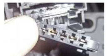
The plug and terminals had become badly corroded.
